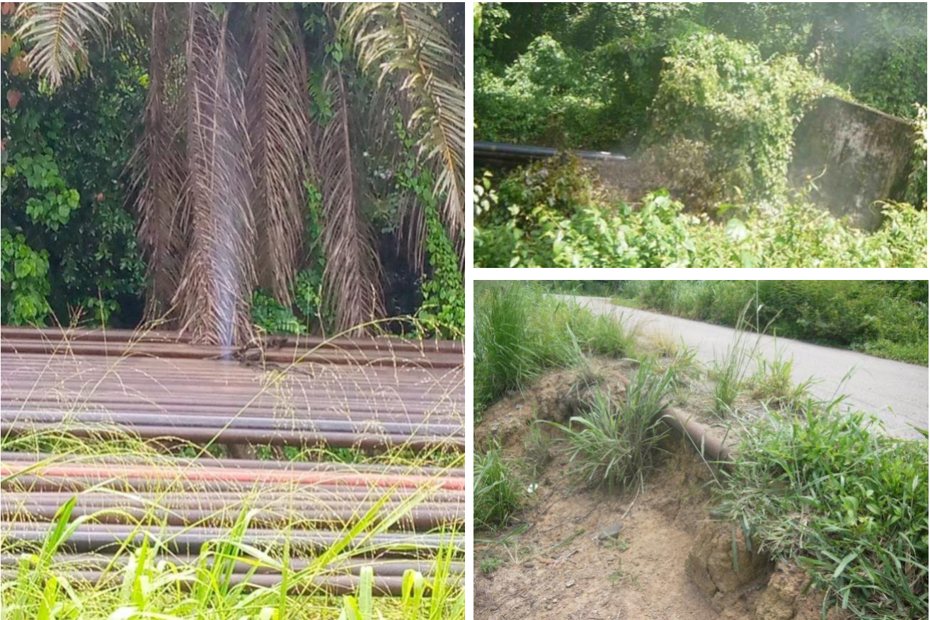
Photo, clockwise starting left: A high pressure gas leak from rusted gas pipelines; Gas pipelines and structure overgrown with plants and leaking gas; Gas pipeline running alongside a road laid by NAOC contractors. (SDN)
