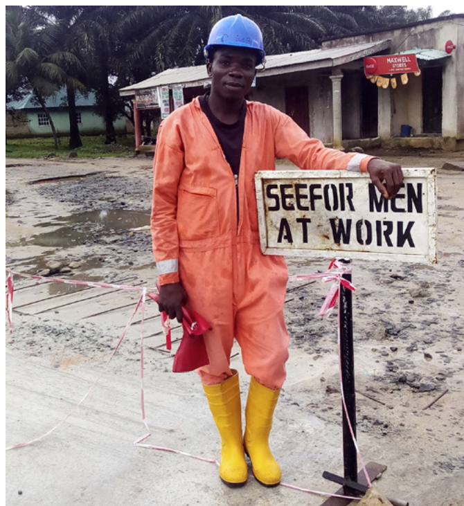
Nonwa's Community Secondary School, pictured here during repairs, was in dire need of renovation
