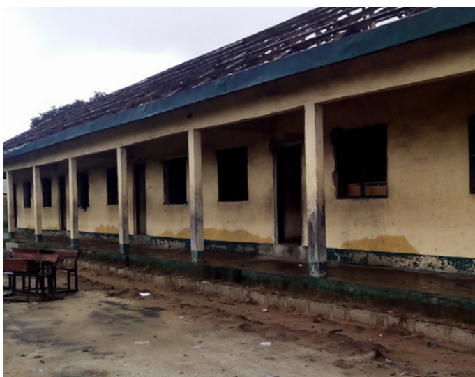
Nonwa's Community Secondary School, pictured here during repairs, was in dire need of renovation
